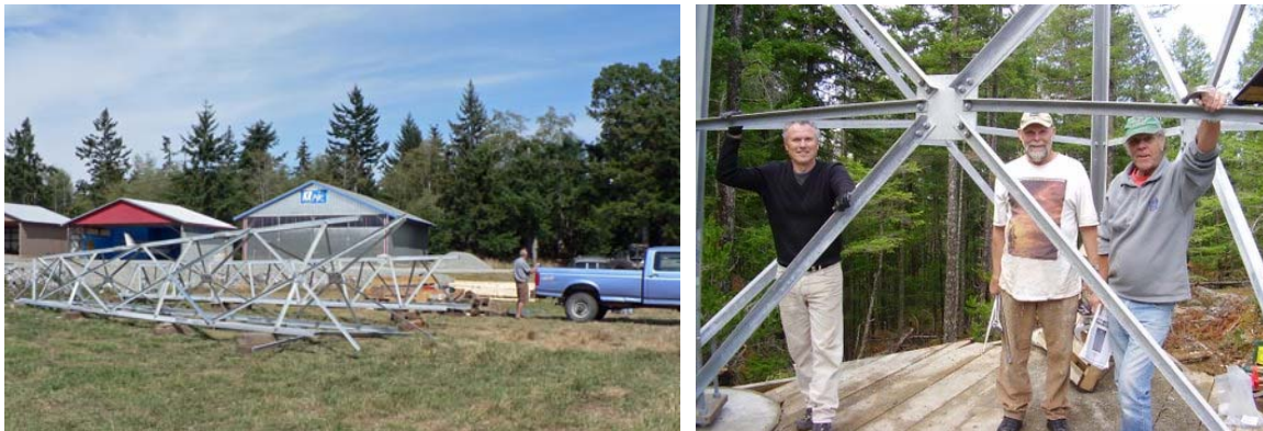
The tower was partially assembled at the Gillies Bay airport; the bottom section was assembled on site.
