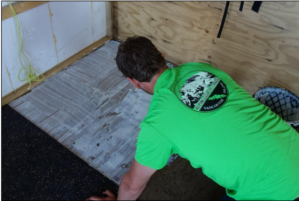
Image 17: After the heli lift volunteers began to install interior finishing items such as rubber flooring.
